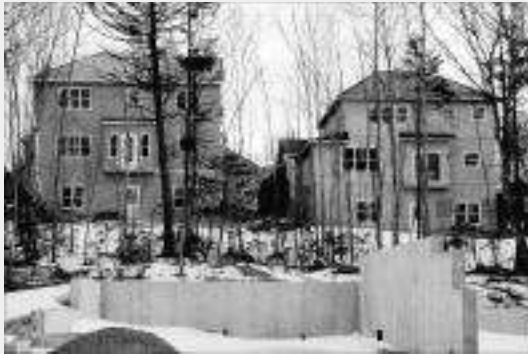
The traditional concrete foundation wall, with no insulation, is disappearing from building sites.
